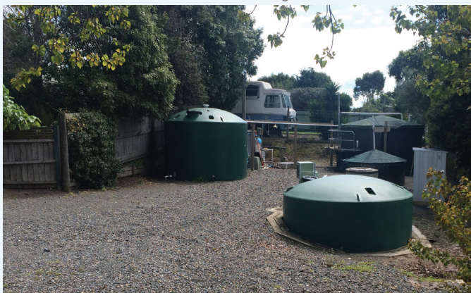
Kingseat Wastewater Treatment Plant.
